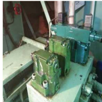
Gambar 3. Control Hidrolis CPP
